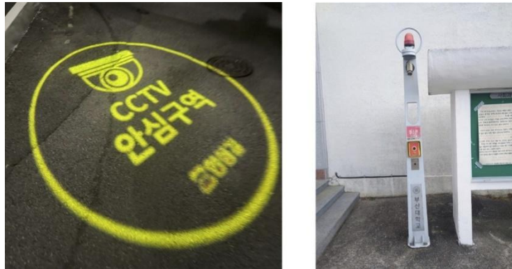
Figure 9: CCTV projections (left) and emergency button with camera (right).
